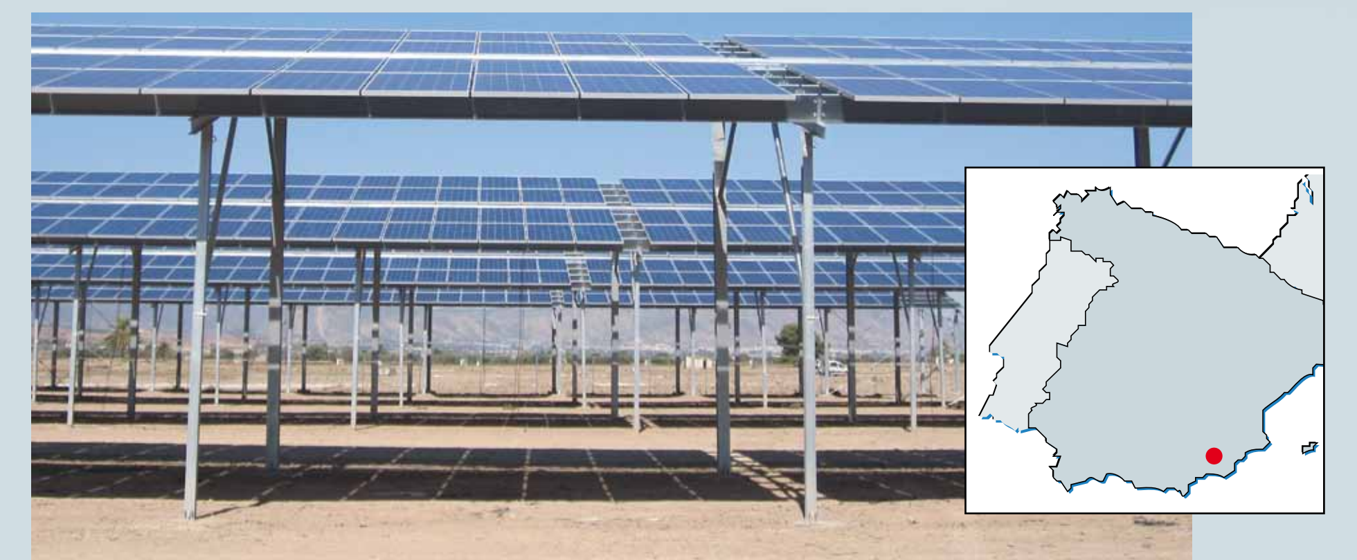
2 MWp system in Murcia, Spain
