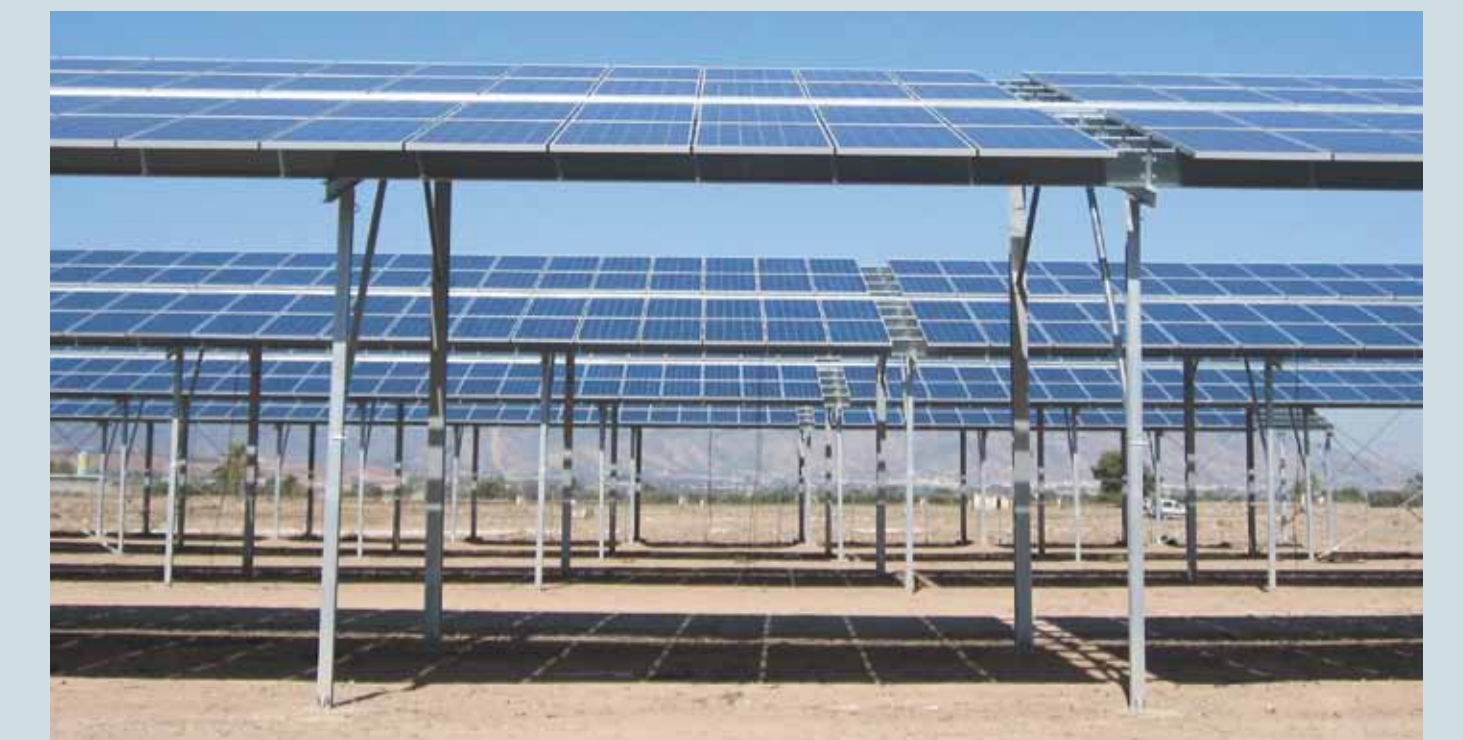
2 MWp system in Murcia, Spain
