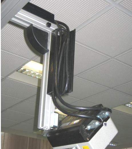
Long cables routed inside the PVC conduit.
