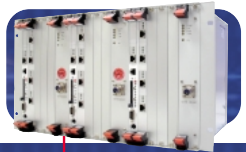
Fully electronic railway control centre (Photo: MEN)
